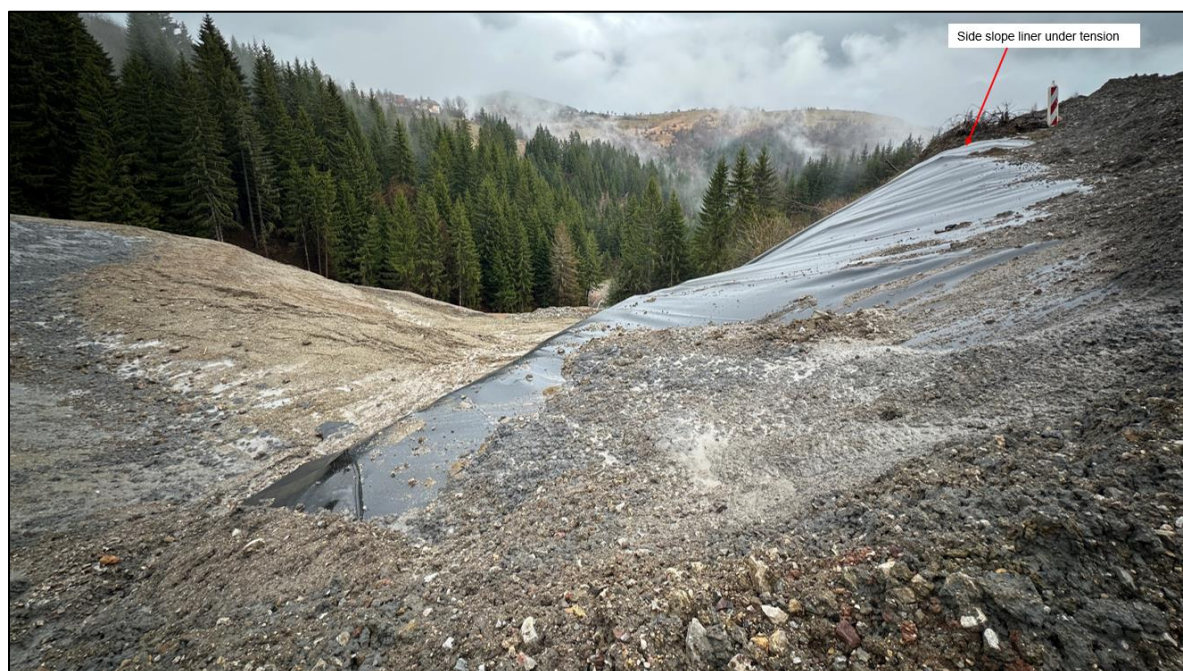
Figure 18-6: Annotated photograph of the Temporary TSF showing side slope HDPE liner under tension (SRK photograph, 25 March 2025)
